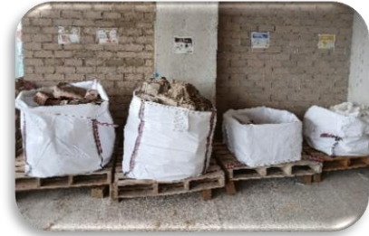
Figure 5: Segregation at construction sites
